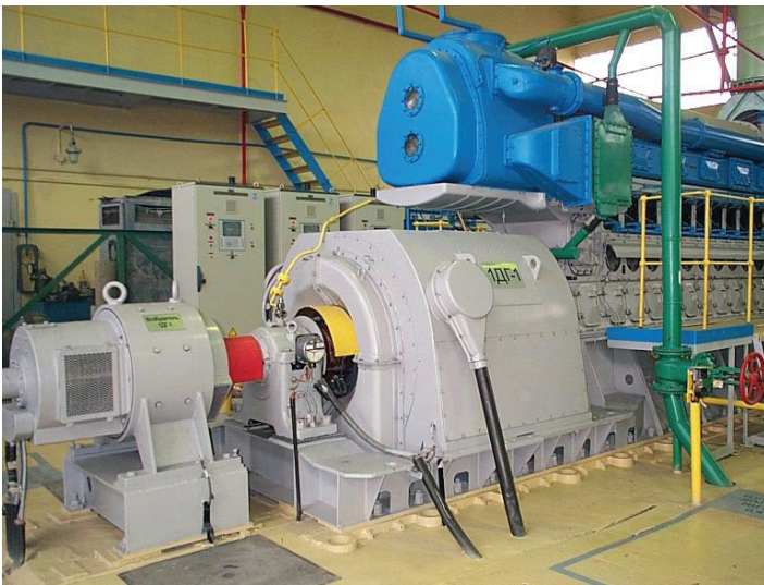
Diesel generator and Diakont control system
