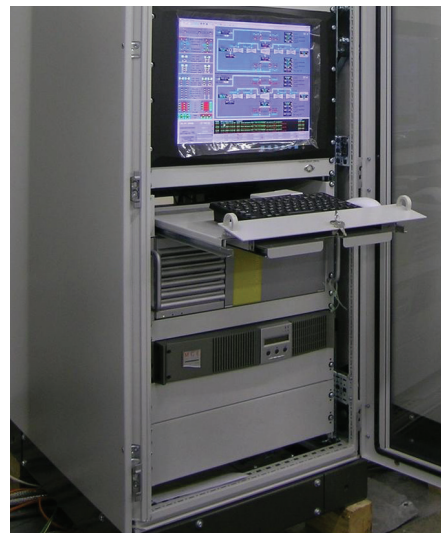
Diesel generator control system interface
