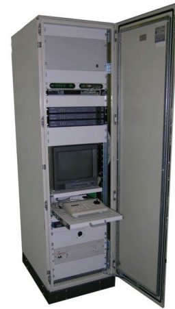
System electronics cabinet
